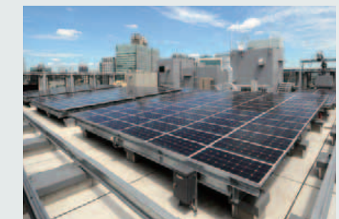
Solar panels at Nittsu Shoji Head Office
