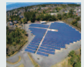
Solar power generation by Nittsu Real Estate (Izunokuni)
