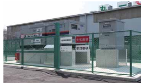
Emergency Power Generator
