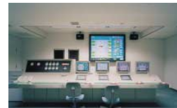
Monitoring equipment in the control room
