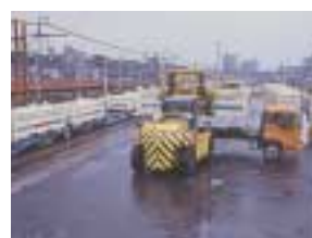
Hauling of surplus soil from construction project at Saitama New Urban Center
